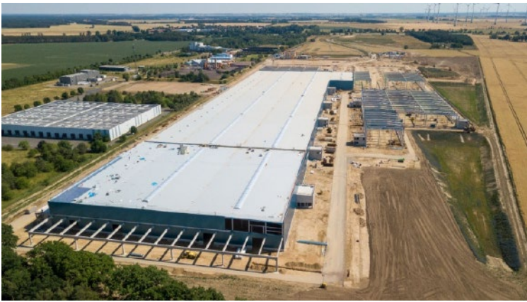
Under construction the new Nokera modular timber framed homes factory in eastern Germany
